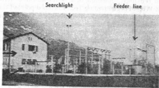
Overall view of a transformer station
